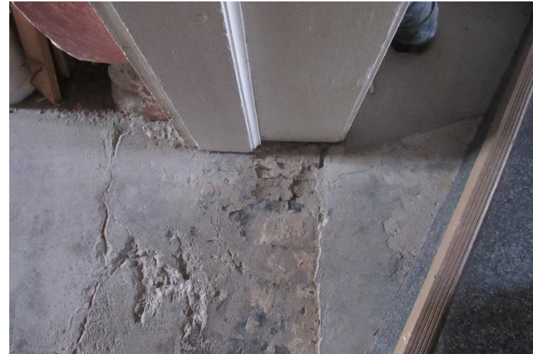
Photo #S2: Cracks and spalling on the SOG.
