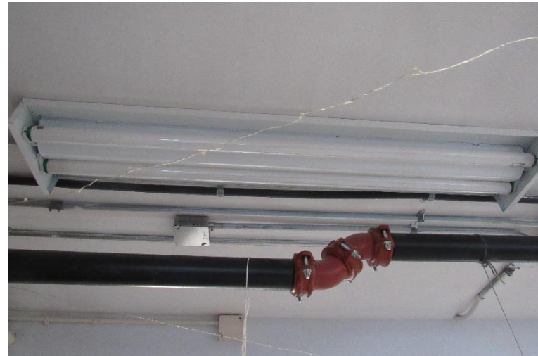
Photo #E6: Typical ceiling-mounted linear fluorescent light fixtures with T12 bulbs.
