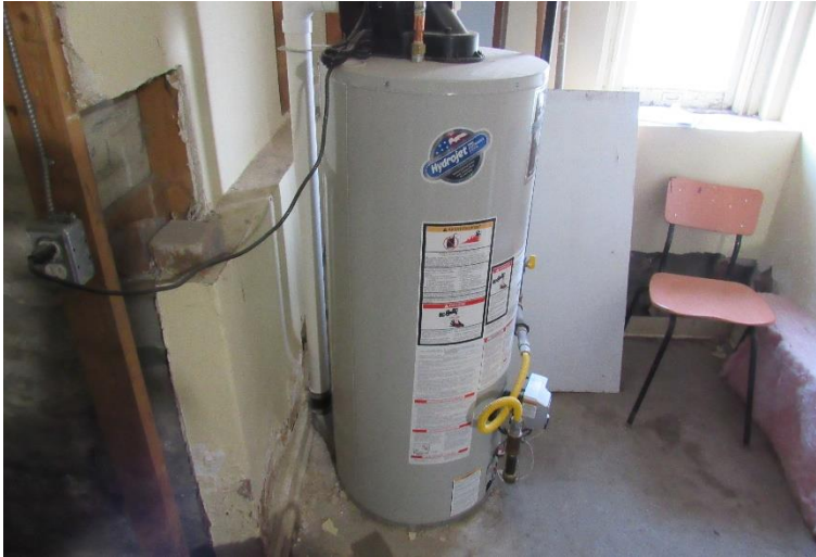
Photo #M3: Gas fired domestic water heater.
