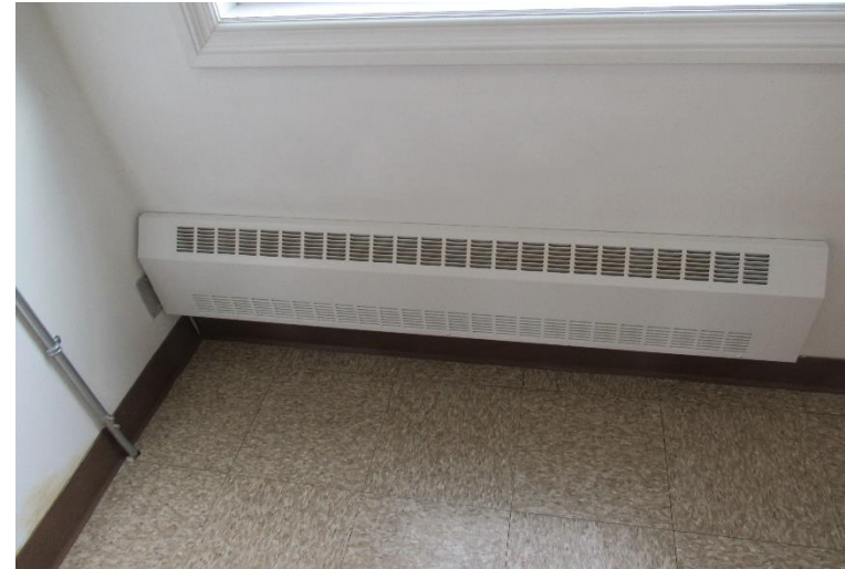
Photo #M6: Typical electric wall heater.
