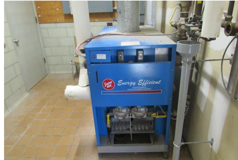
Photo #M4: Gas fired boiler.
