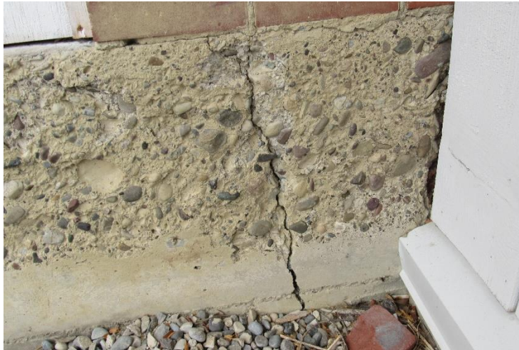
Photo #S1: Crack on foundation wall.
