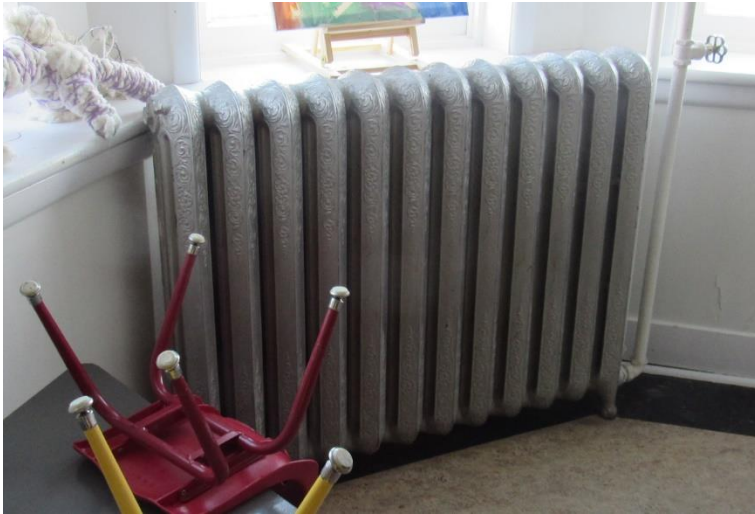
Photo #M5: Typical original hydronic radiant wall heater.
